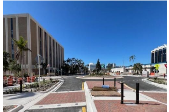
The new roundabout located at Ringling & Pine with the County Admin Building on the left, and U.S. Post Office on the right. It is scheduled to open this spring.
