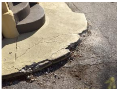
Turning Vehicles Curb Damage, NE Corner Cherry Lane and Rawls Avenue
