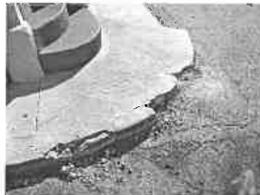
Turning Vehicles Curb Damage, NE Corner Cherry Lane and Rawls Avenue
