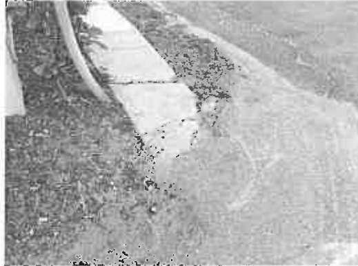
Turning Vehicle Curb Damage SE Corner Cherry Lane & Rawls Avenue
